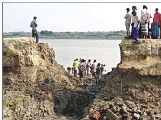
Locals trying to repair the breached portion of the embankment on Kholpetua River at Puijala in Sreeula union of Assassuni upazila under Satkhira district yesterday as the breach left about 5,000 people marooned in adjacent areas. Photo: STAR
