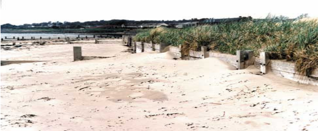
Timber breastwork functioning successfully within an estuary.
